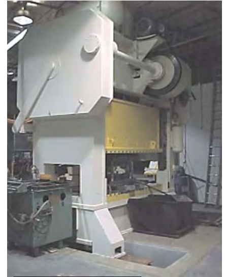
Press mounted on SVS spring isolators.
