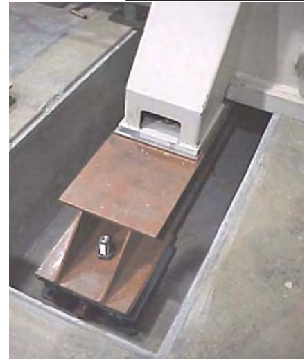
Close-up of an isolator and outrigger beam under a press foot.
